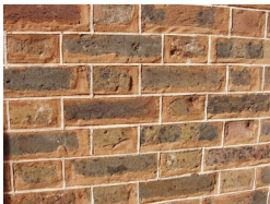
Mortar needs repair
